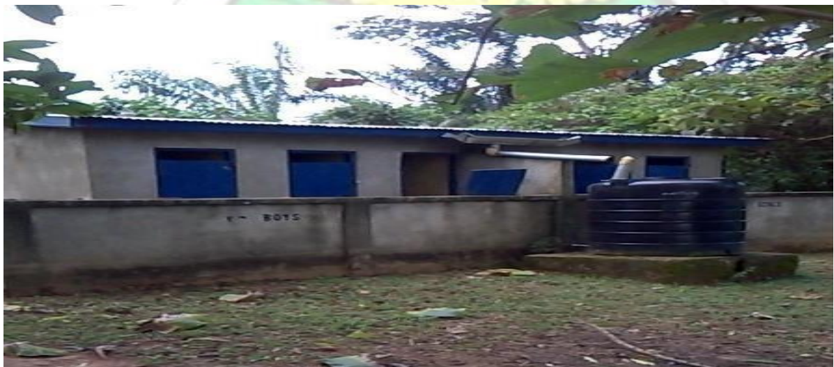
Figure 4.6 Broken doors to toilet facility at St Anthonys Basic
