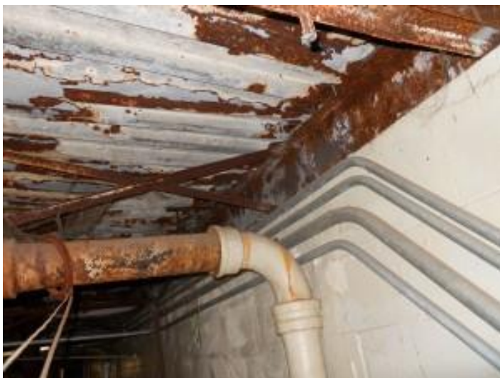
Fig 2.6 Special requirements failure
