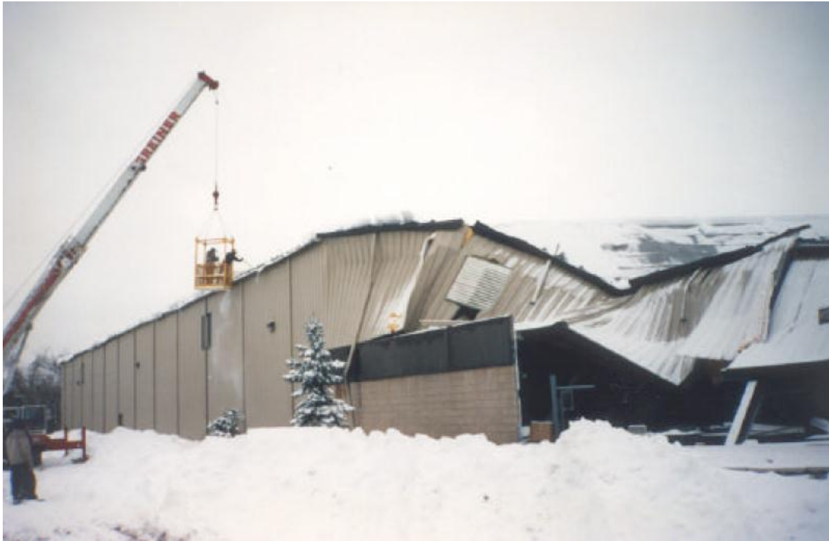
Fig. 2.3 Ultimate Failure of Roofs
