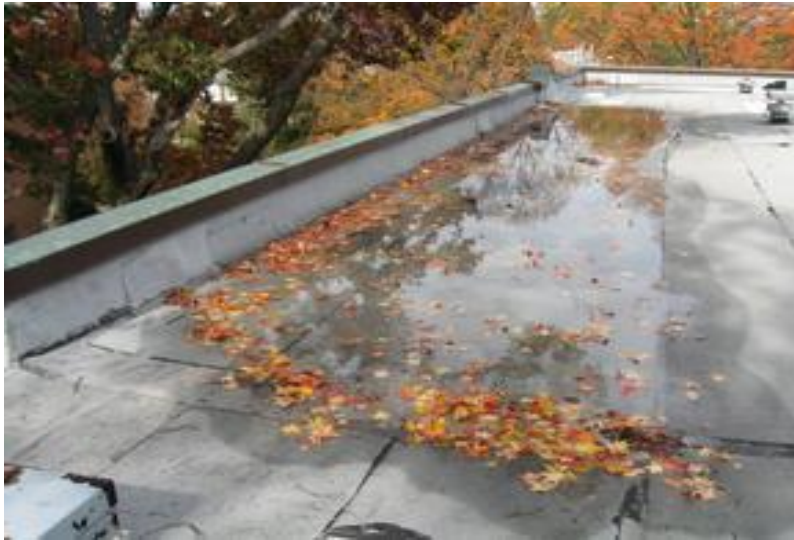
Fig 2.4 Serviceability Failure of Roofs
