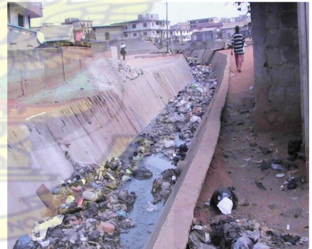
PLATE 4 Gutter filled with waste
