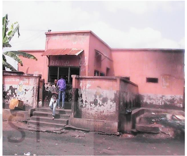
PLATE 6 Poorly maintained KVIP
