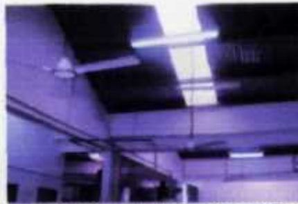
Figure 66. Lighting System in the Production Area (Source Papso Ghana, Ltd – Off Spintex Road Accra)
