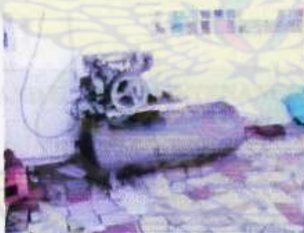
Figure30. Air Compressor (Source: Nourisher Processing Ltd Accra - North)
