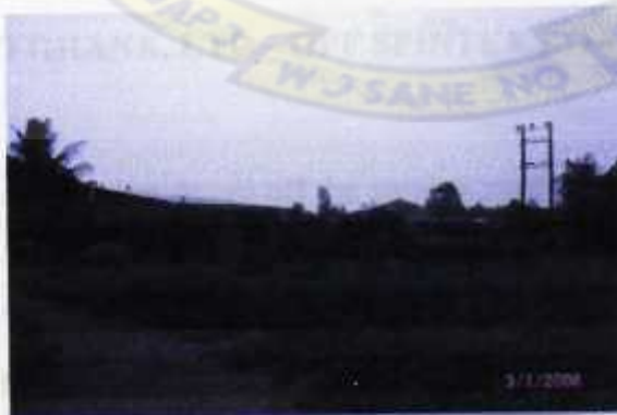
Figure 45. Power Supply To The Factory (Source: Bomarts Farms Limited – Nsawam)
