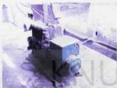
Figure26. Standby Generator (Source: Nourisher Processing Ltd Accra - North) The standby generator is also located behind the production block and it is used when the power from the electricity company of Ghana is off to give power for the operation of the company.
