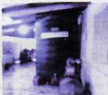
Figure28. Water Storage Tank (Source: Nourisher Processing Ltd Accra - North)
