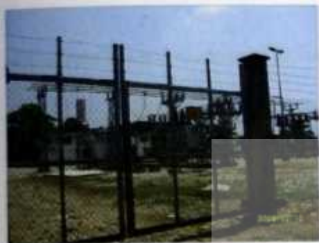
A PICTURE OF PRIMARY SUB-STATION E LOCATED AT THE SUAME MAGAZINE. IT'S THE ONLY STATION DISTRIBUTING POWER TO THE FIVE TRANSFORMERS AT THE MAGAZINE.
