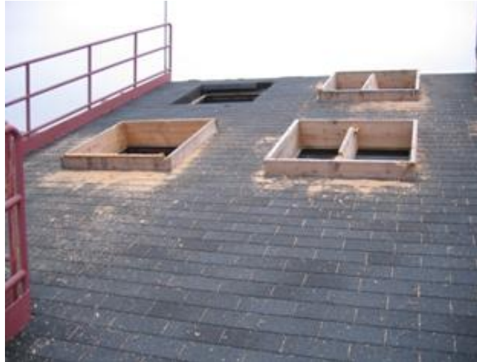
Figure 2.2: Roof of burn building with removable ventilation panels (Source: Berks County Fire Training Centre, 2008)
