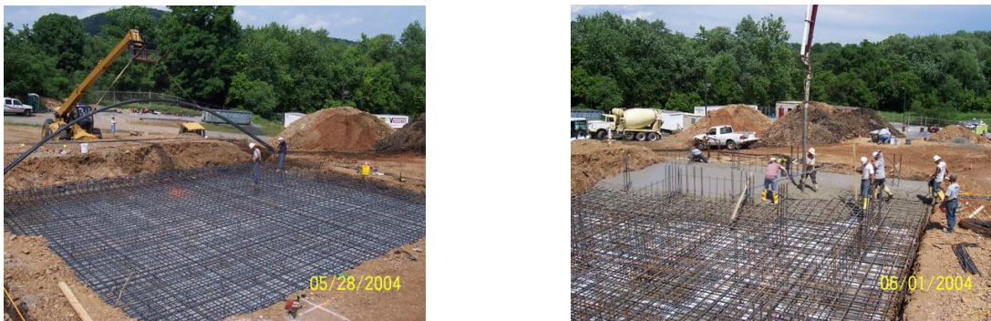
Figure 2.18: Steel framework for the foundation of the burn building (Source: Berks County Fire Training Centre, 2008)
