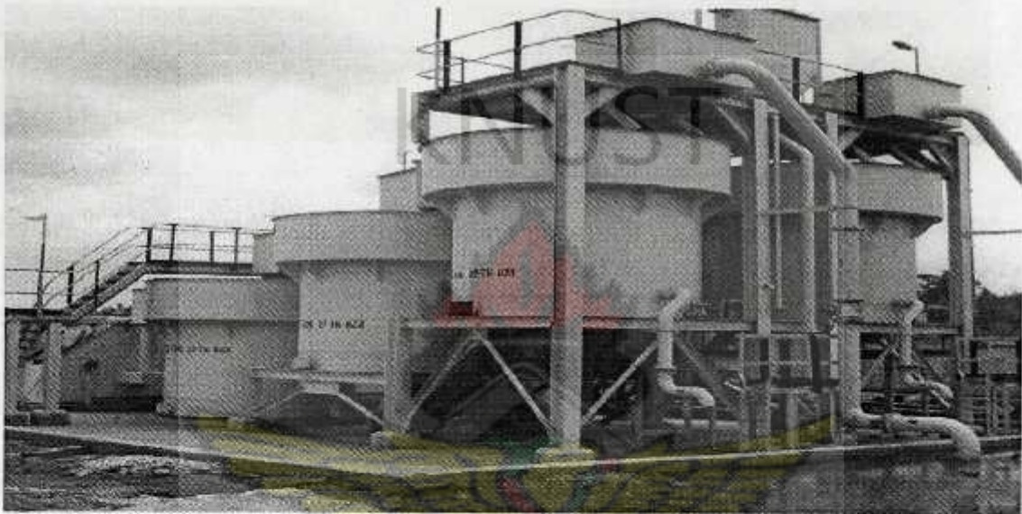
Figure 3-4: CIS holding tanks
