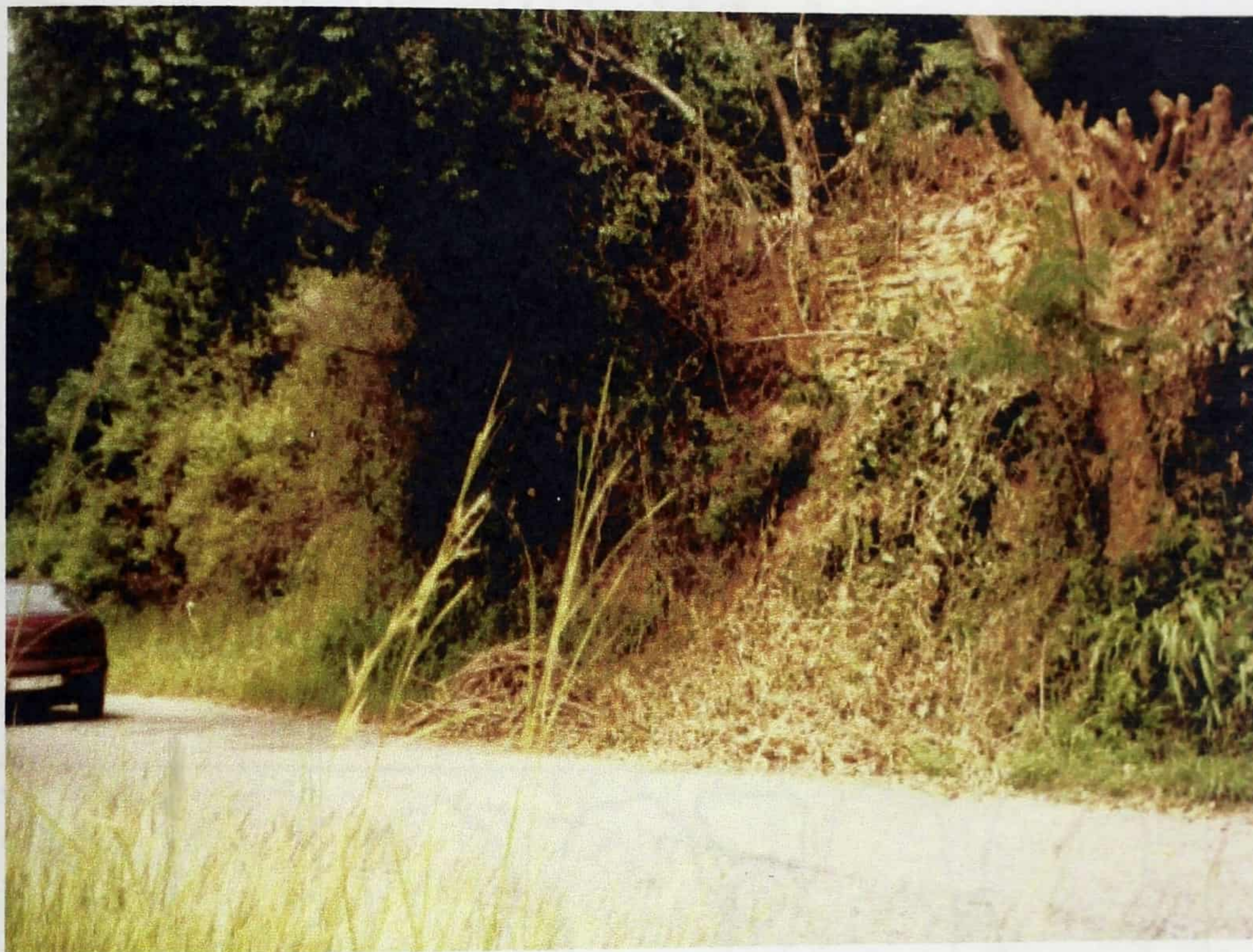
Plate 7: Un-coursed random rubble pitching along Larteh-Ayikoma road
