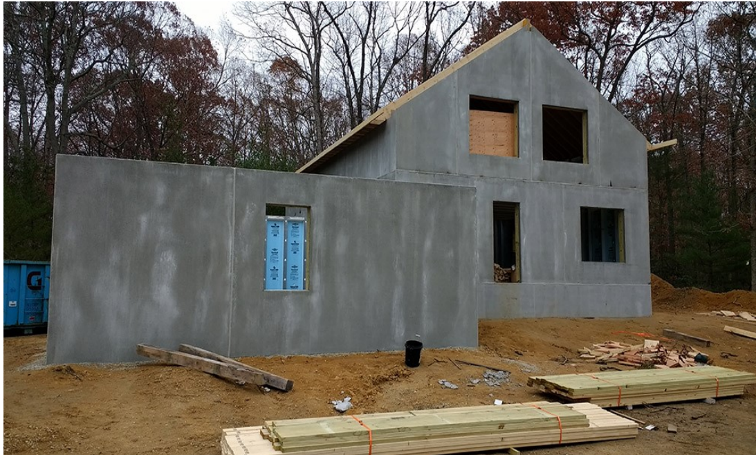
Plate 2.7: Massive Wall System with prefabricated concrete panels or Using Cement Foam Panel
