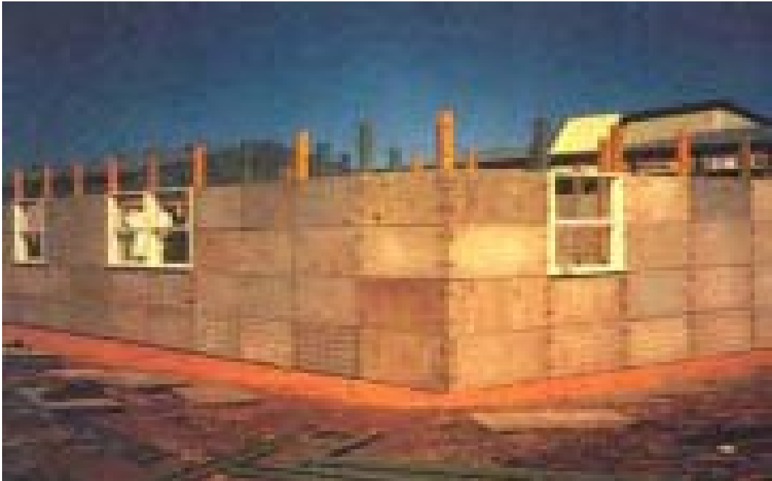
Plate 2.9: Metal Pole Frame or Steel columns with Concrete Panels as an example of load bearing framework
