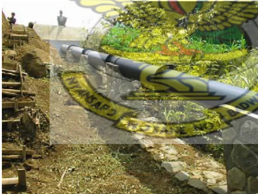
Figure 2.8: Mild Steel Penstock
