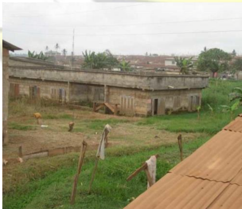
Plate 12: Uncompleted building on wetland area
