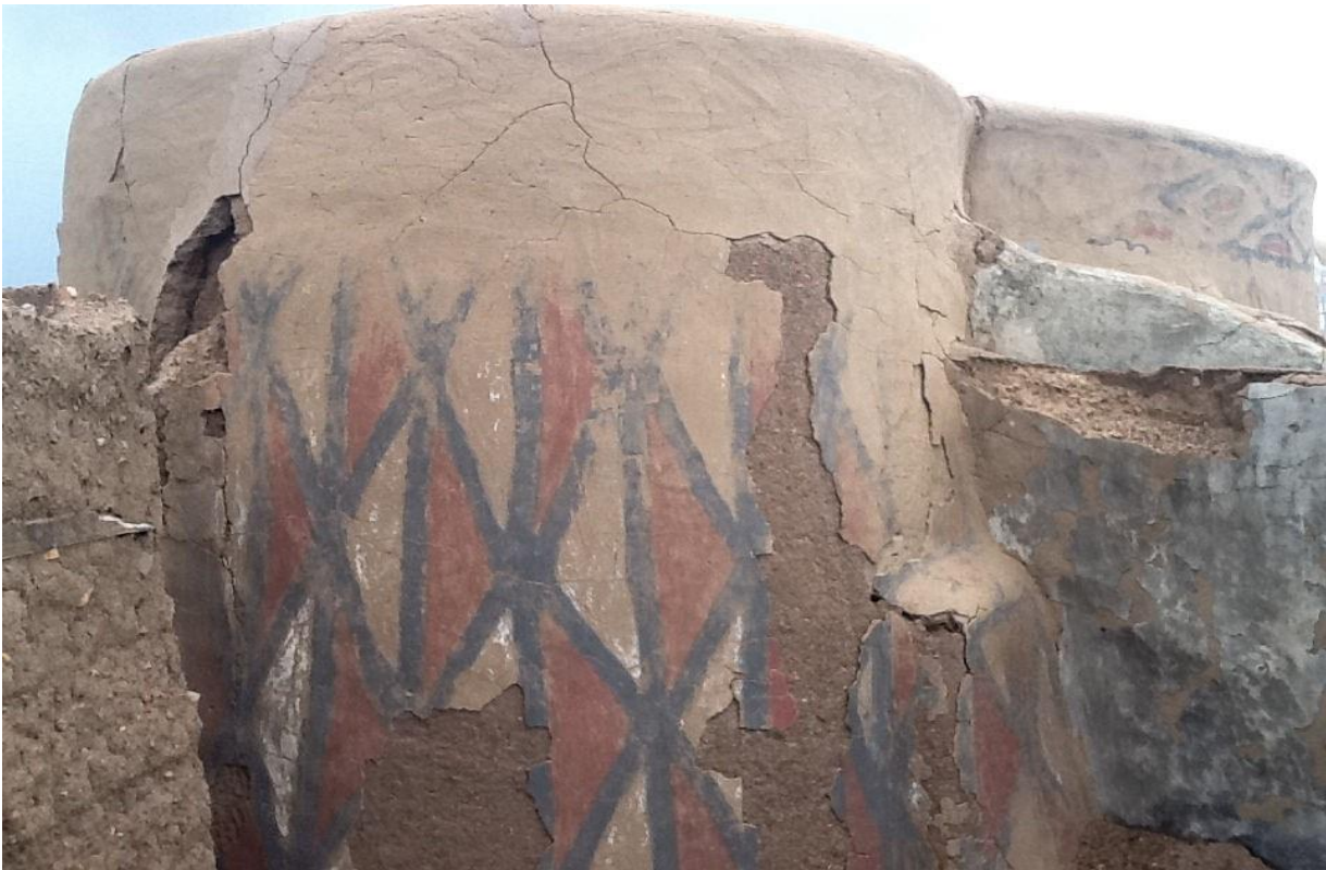
Plate 4.60: A Sirigu building crying for refurbishment. Source: Photographed by Researcher.
