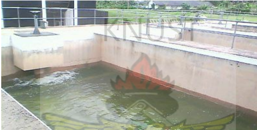
Figure 3.6 One of the six rapid sand filters at the treatment plant
