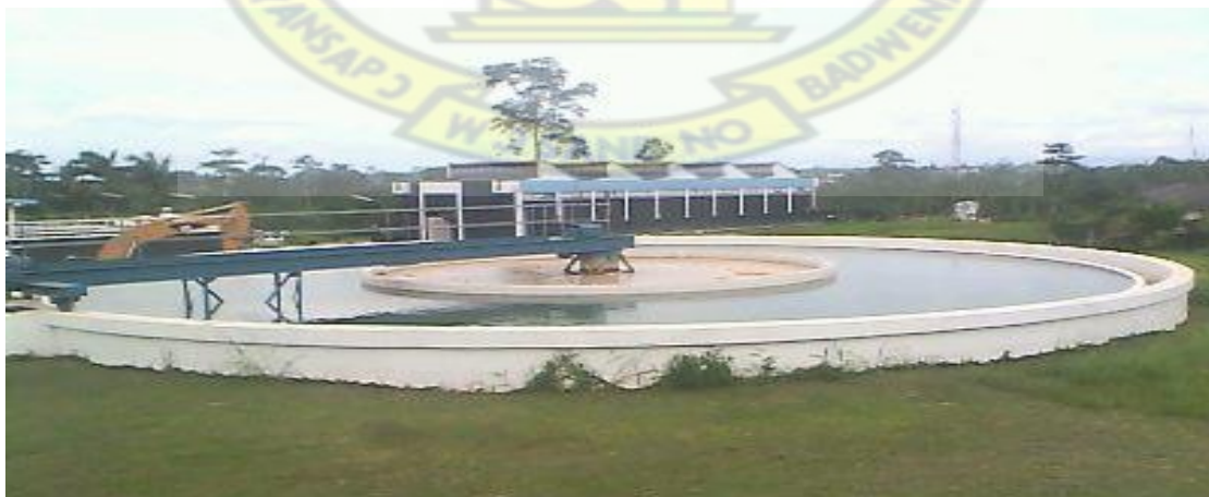
Figure 3.5 Clarifier showing the sedimentation chamber of the Daboase Water Treatment Plant
