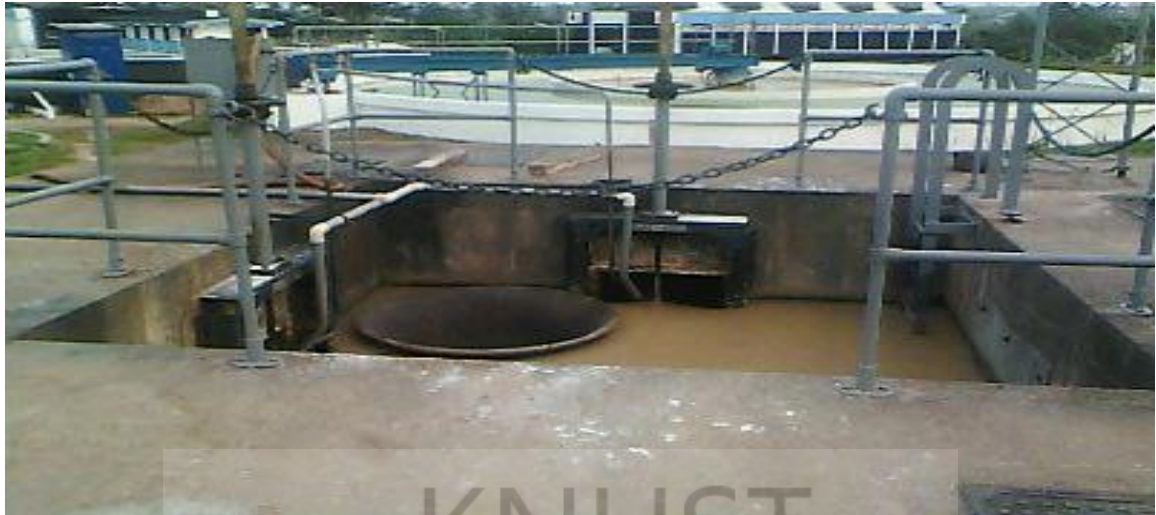
Figure 3.4 Coagulation chamber of the Daboase Water Treatment Plant
