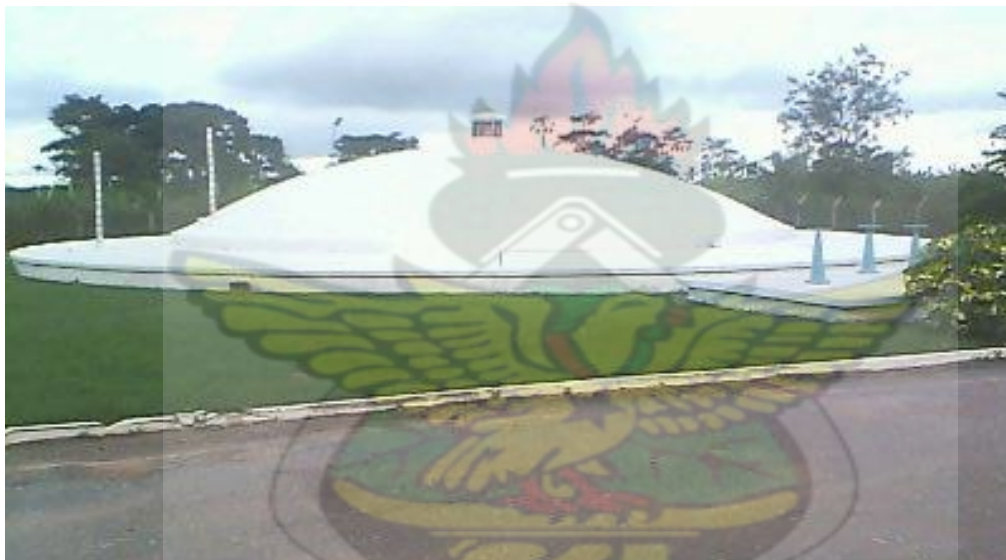
Figure 3.7 Underground water storage well of the Daboase Water Treatment Plant
