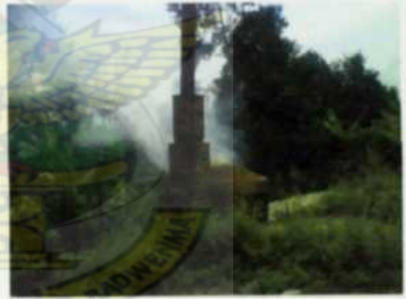
Fig6. incinerator for handling solid waste
