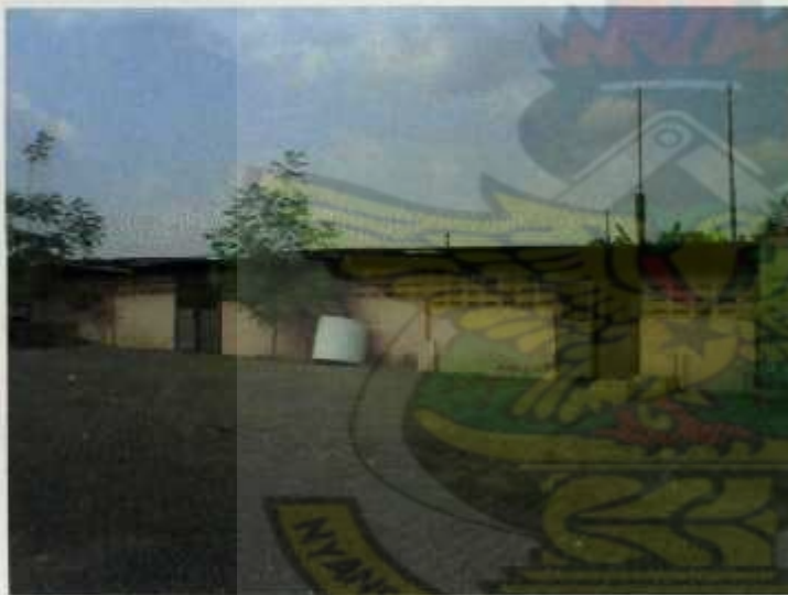
Fig8. Boiling room with its concrete columns and honey combs
