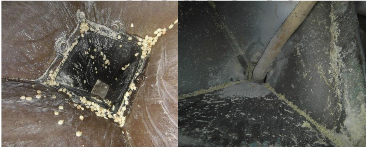
Plate 9: Discontinuous welding of the hopper creating dead areas
