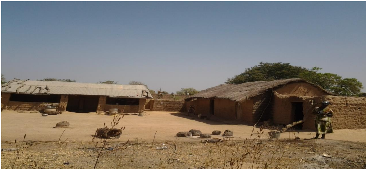
Figure: 4.7 A house in Guri with infrastructural problems, a study community in Zone 4, 2016
