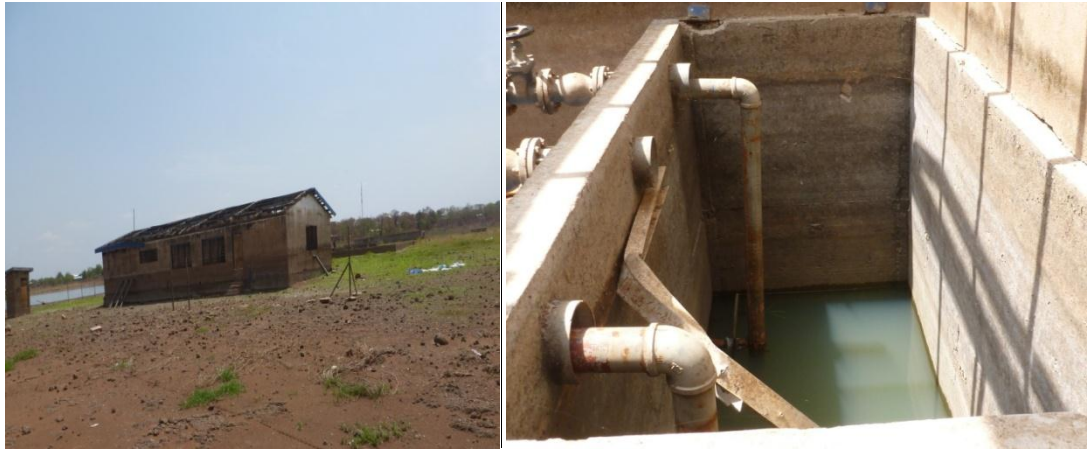
Figure 2-6: Abandoned STWSS Facility due to the 2010 Floods.
