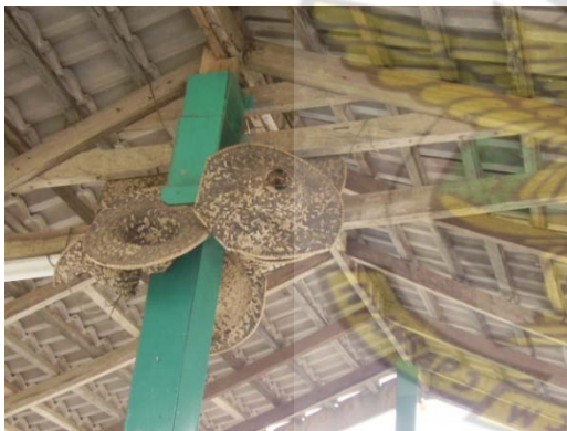
Figure 4.11: Straw hat lighting
