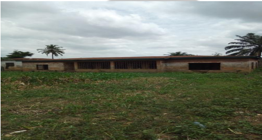
Plate 7.3: Abandoned houses due to floods (Atonso S-line) Source: Fieldwork (2017)
