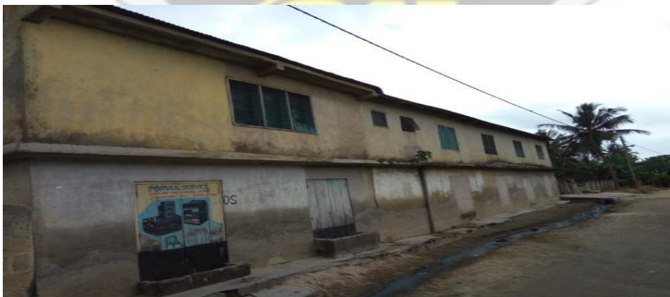
Plate 8.6: Disserted ground floor due to floods. See the level of flood water on the building (Breman) Source: Fieldwork (2017)
