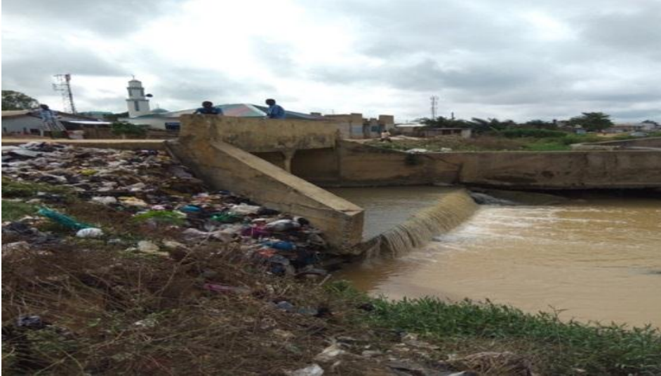
Plate 5.3: Waste-laden storm drain (Kwadaso) Source: Fieldwork (2017)
