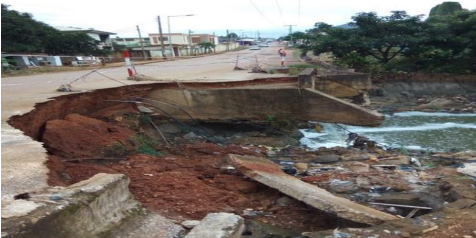
Plate. 5.6: Stream erosion-induced Collapse Bridge (Kwadaso)
