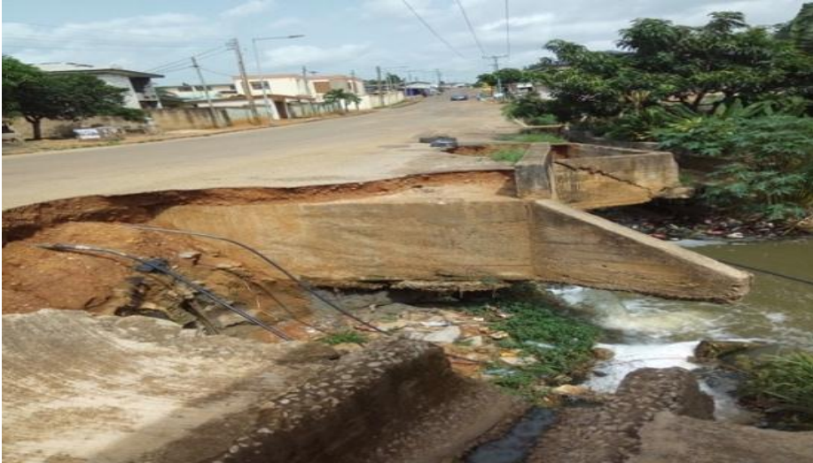
Plate5.5: Undermined bridge (Kwadaso)
