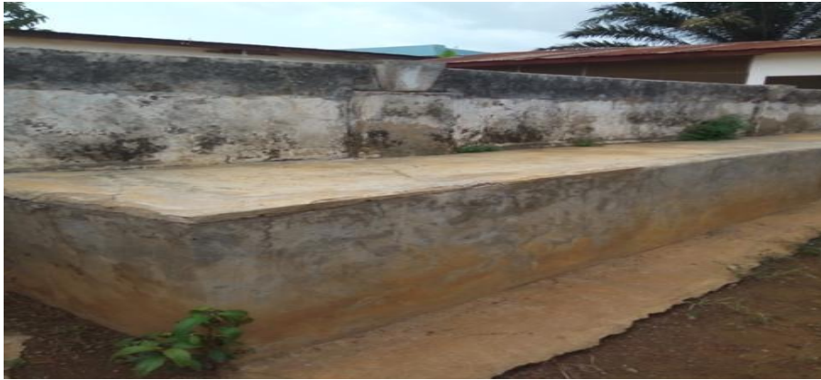
Plate 8.1: Massive flood defence wall (Kwadaso) Source: Fieldwork (2017)
