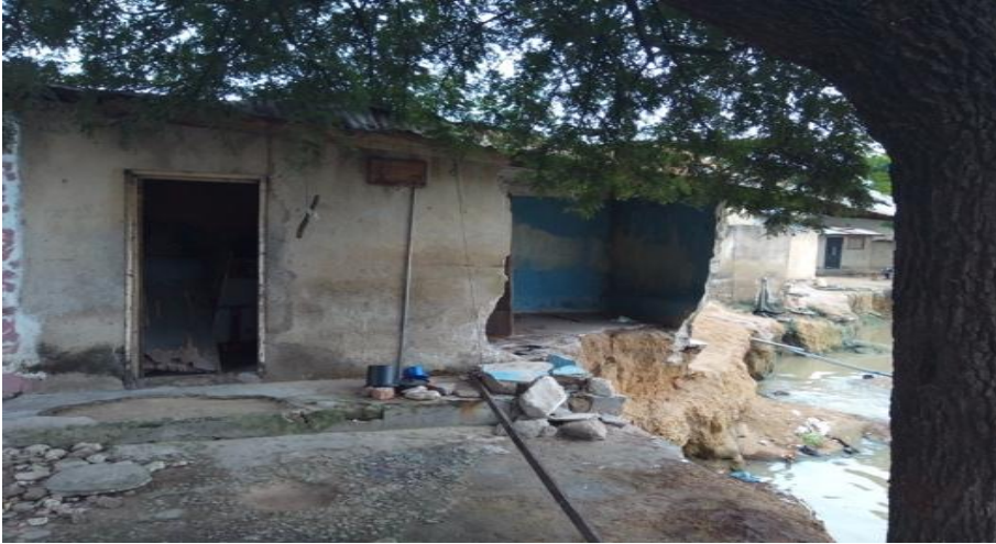
Plate 7.6: Flood-induced undermined building (Ayigya Zongo) Source: Fieldwork (2017)
