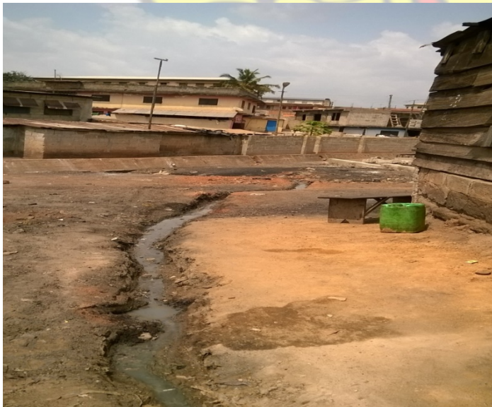
Plate 6: Poor state of Drains in Parts of Aboabo
