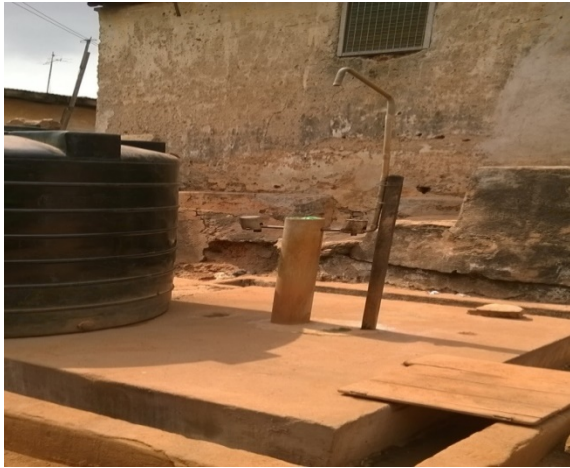
Plate 1: Exposed Foundation of a building at Aboabo
