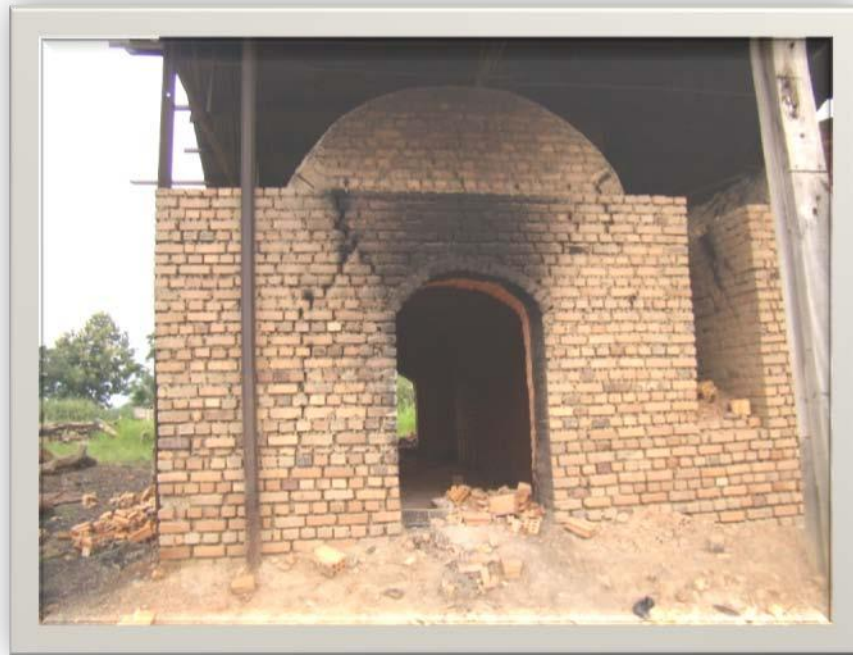
Plate 4.14 Cracks on a kiln at Tanoso
