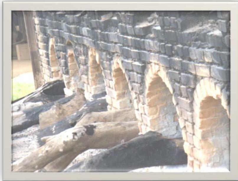
Plate 4.15 Firebox of a clamp kiln
