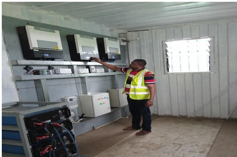
Figure 12. Configured AMI control station (Source: Authors Construct, 2023).
