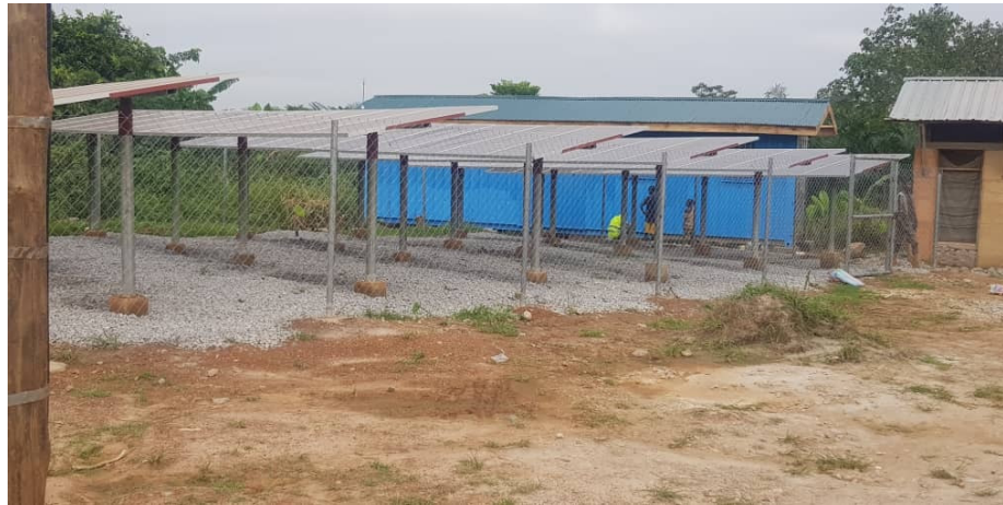
Figure 10. Implemented solar PV farm in Yeboahkrom (Source: Authors Construct, 2023).
