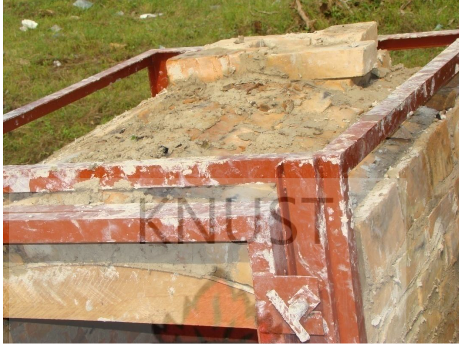
Plate 3.46 The dome of the kiln
