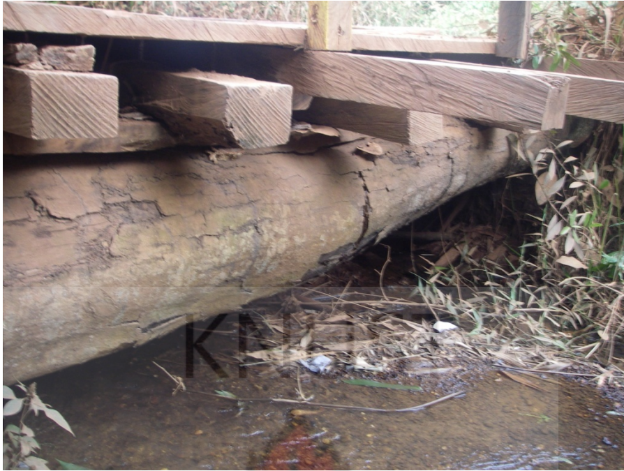
Plate 4a The old bridge on the Chira River in the CGML Concession Area
