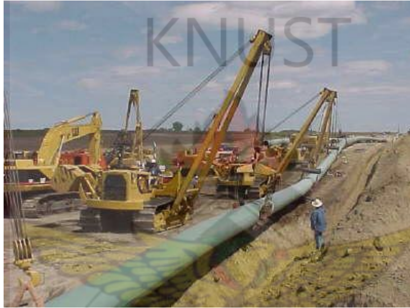
Figure 3.2 Crew Lowering a Pipeline into a Trench (Source: Photo courtesy of U.S. Pipeline)
