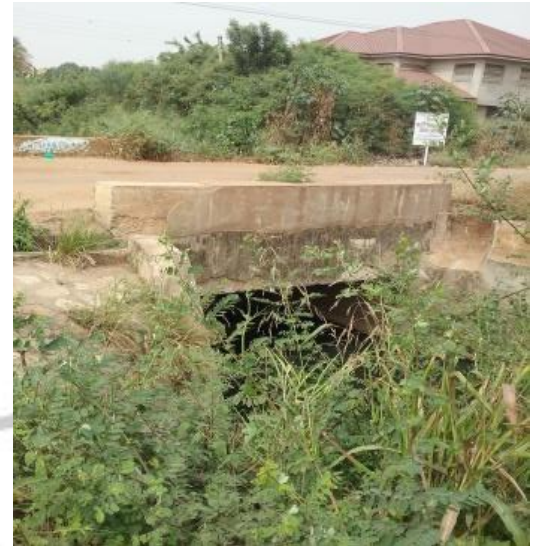
Plate 2.5A: Section of road showing a lot of defect on Jasmine Street at Community 20, Tema. Plate 2.5B: This culvert's inadequacy is largely responsible for the defects on the Jasmine Street above.
